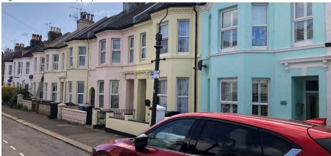
Figure 6: Photo of inappropriate PVCu casement windows
